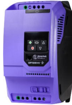
7.5HP VFD for 60GPM Pump Indoor
